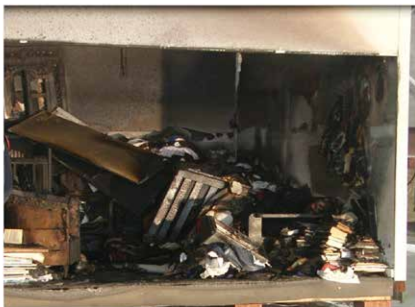
Figure 15: Post fire damage and debris (Test 2)
